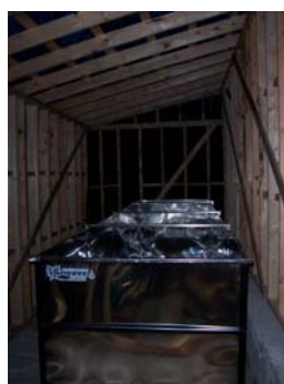
New Stainless Steel Tank in New Building
